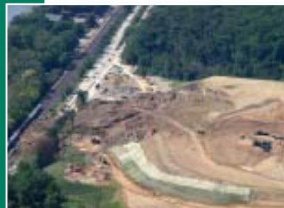
Disturbing slide prone Pittsburgh Red Beds and altering the hydrology of this site are two possible causes of the Kilbuck landslide.
